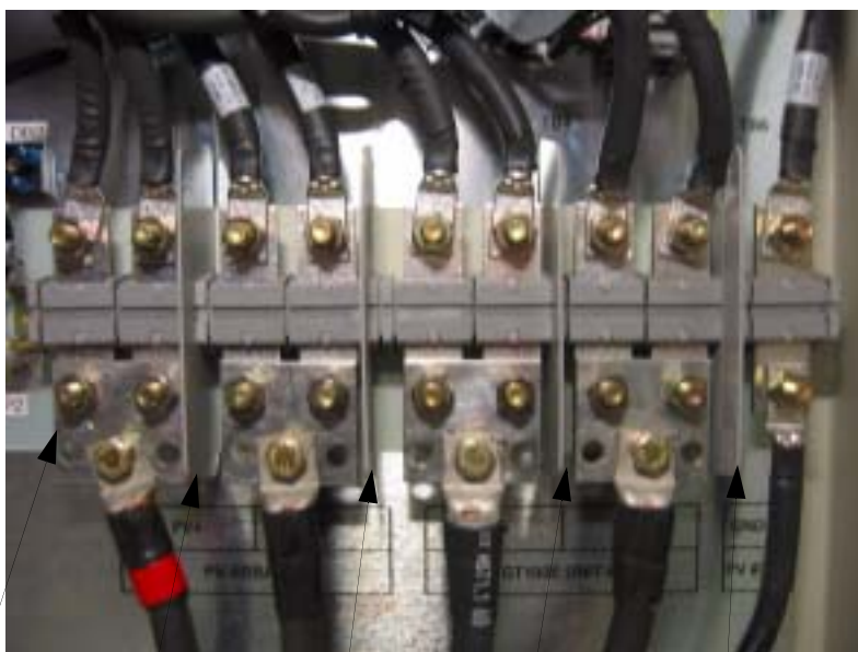
Combiner Box PV ARRAY #2 PV (+) Terminal Combiner Box PV ARRAY #2 PV (-) Terminal Combiner Box GT100E #2 PV (+) Terminal Combiner Box GT100E #2 PV (-) Terminal Combiner Box PV ARRAY #2 GND Terminal
